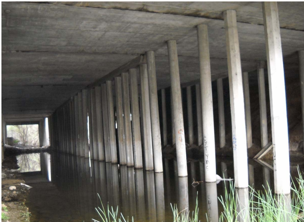
DOWNSTREAM & UPSTREAM EXTENT OF REACH NO. 35, BENEATH U.S. HWY 101 BRIDGE 8 FT. UPSTREAM OF HEC-RAS RIVER STATION 22+92, UPSTREAM DIRECTION
