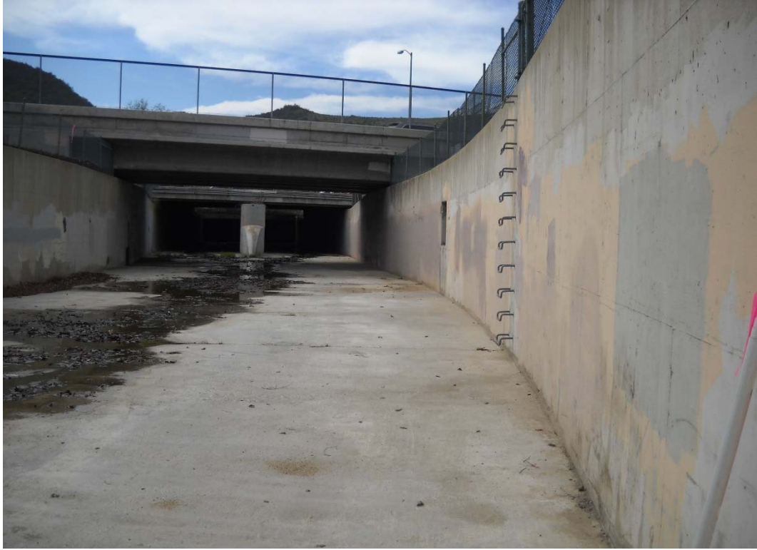
HEC-RAS RIVER STATION 00+16, DOWNSTREAM DIRECTION (CANWOOD ST. BRIDGE AND U.S. HWY 101 BRIDGE)
