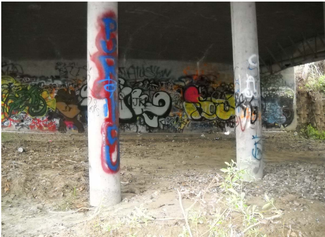
11 FT. DOWNSTREAM OF HEC-RAS RIVER STATION 32+61, LEFT BANK (BENEATH OAK CREEK LN. BRIDGE)
