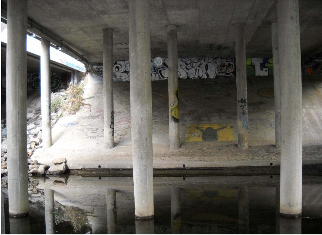
40 FT. UPSTREAM OF HEC-RAS RIVER STATION 25+35, RIGHT BANK (BENEATH CANWOOD ST. BRIDGE)
