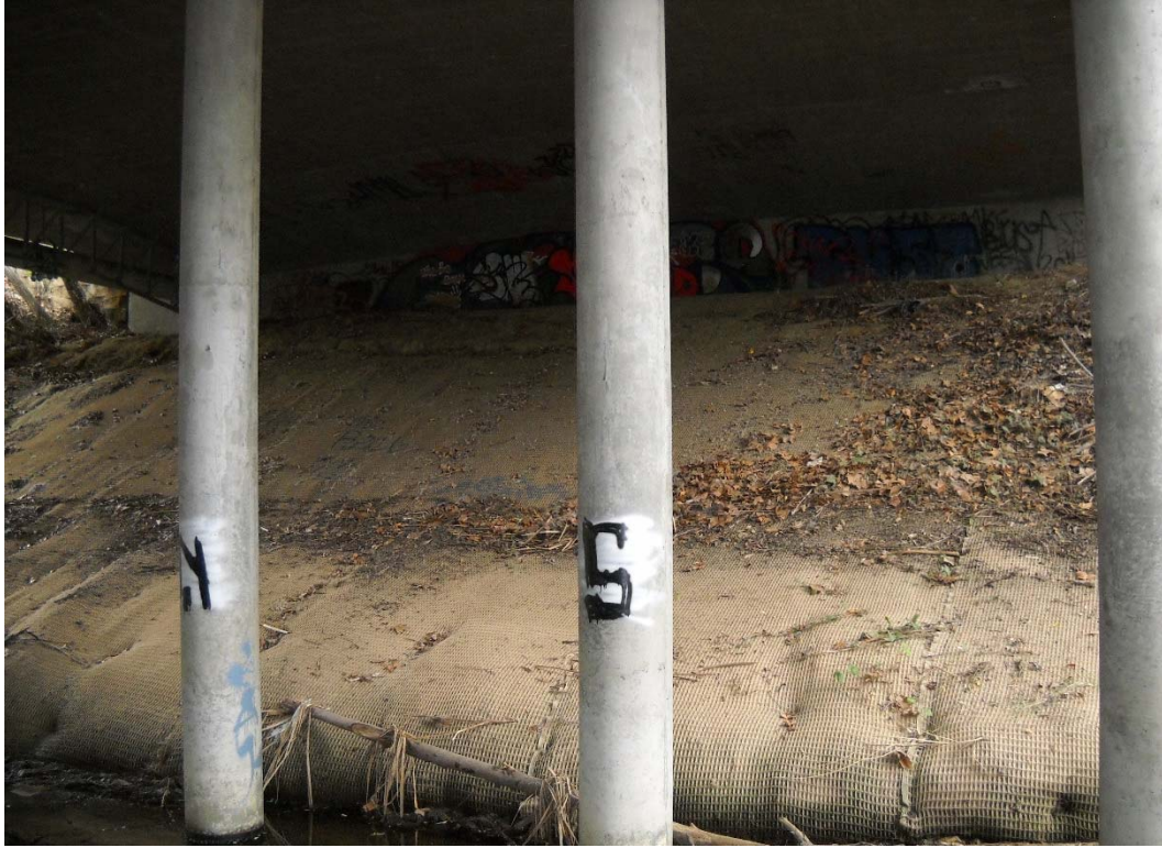
11 FT. DOWNSTREAM OF HEC-RAS RIVER STATION 32+61, RIGHT BANK (BENEATH OAK CREEK LN. BRIDGE)
